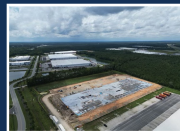
PORTSIDE DISTRIBUTION ±203,000 SF
