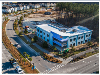
HOME TELECOM HEADQUARTERS OFFICE 20,000 SF Class A office currently under construction and scheduled to deliver in May 2020.
